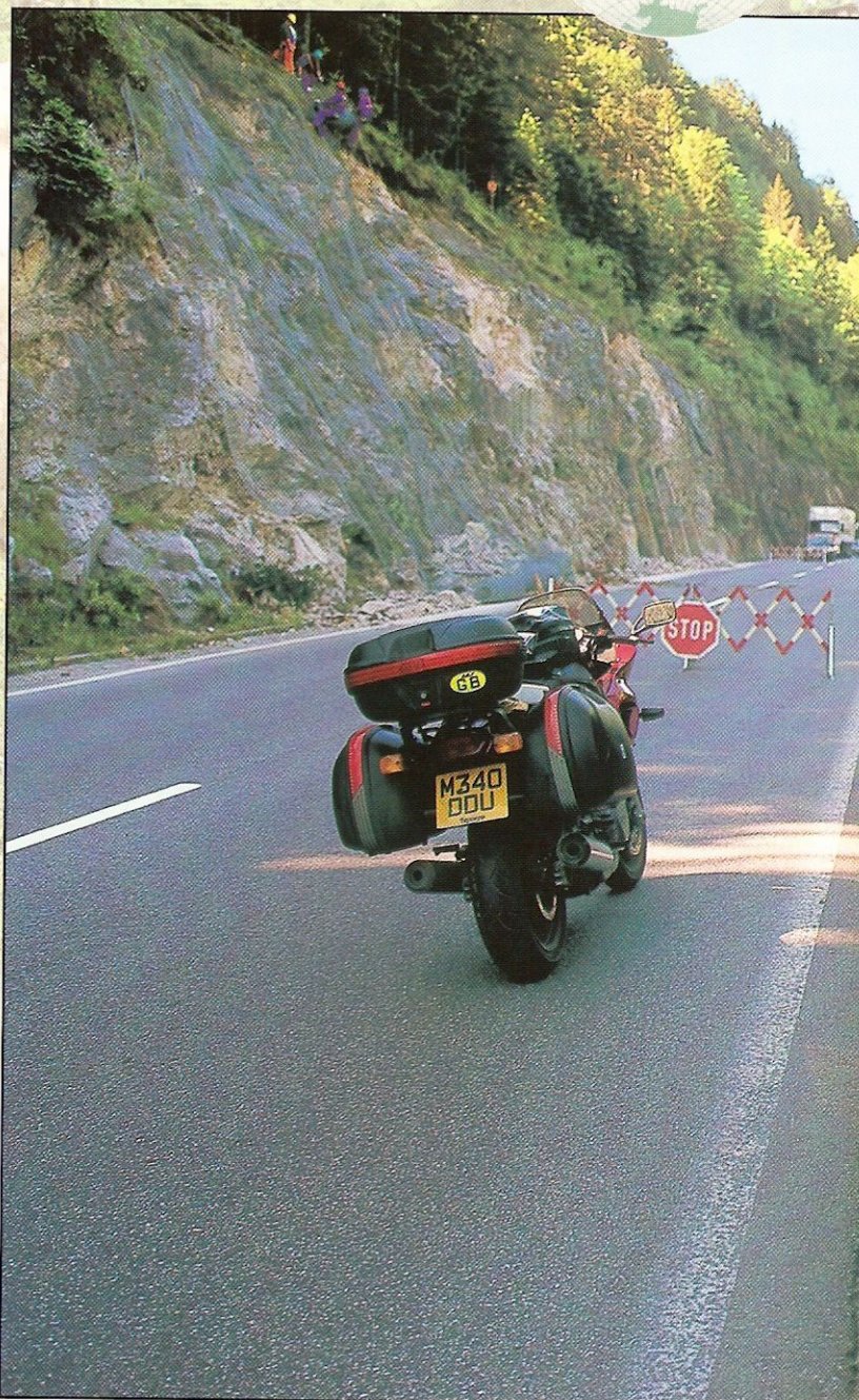
Road works in Switzerland can often mean a delay of half an hour or more. The record was from eleven in the morning until six at night!
